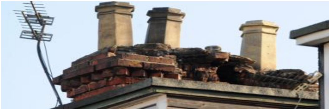
A chimney stack on a house in Goole, East Yorkshire, that was damaged by the earthquake
